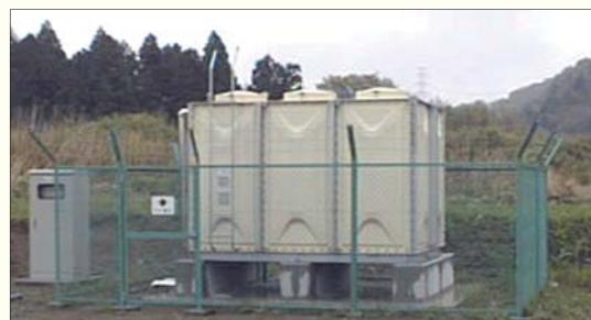
Contaminated water recovery equipment installed at former industrial waste landfill site
